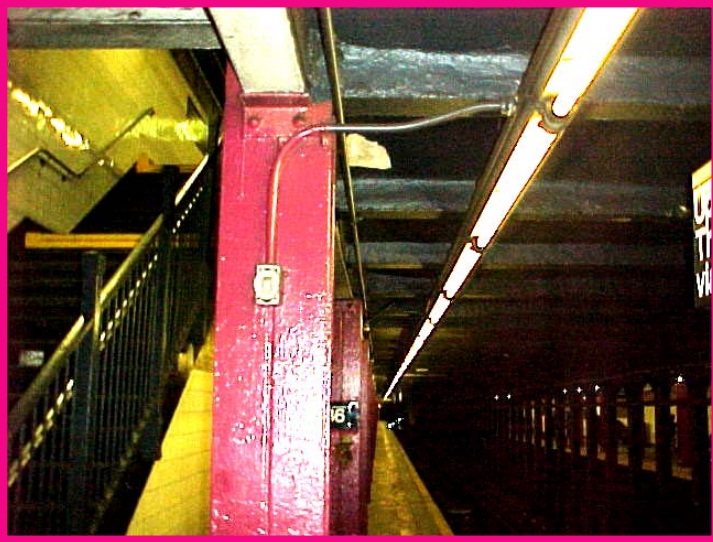
Typical NYCT Station Lighting Interface
